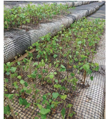
Figure 6 offers a close-up look at the plants growing out of the geogrid reinforced bio-engineered slope.
