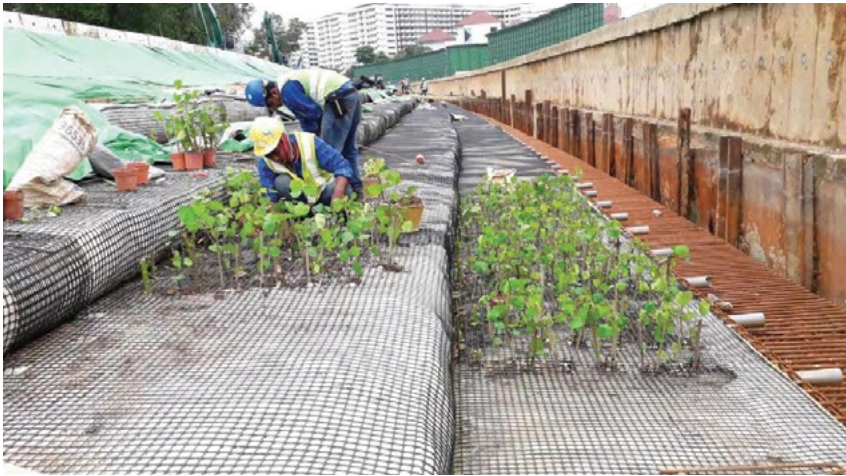
Figure 5: Geogrid-geotextile combination facing that has been completed for the project, with plants starting to grow on it.
