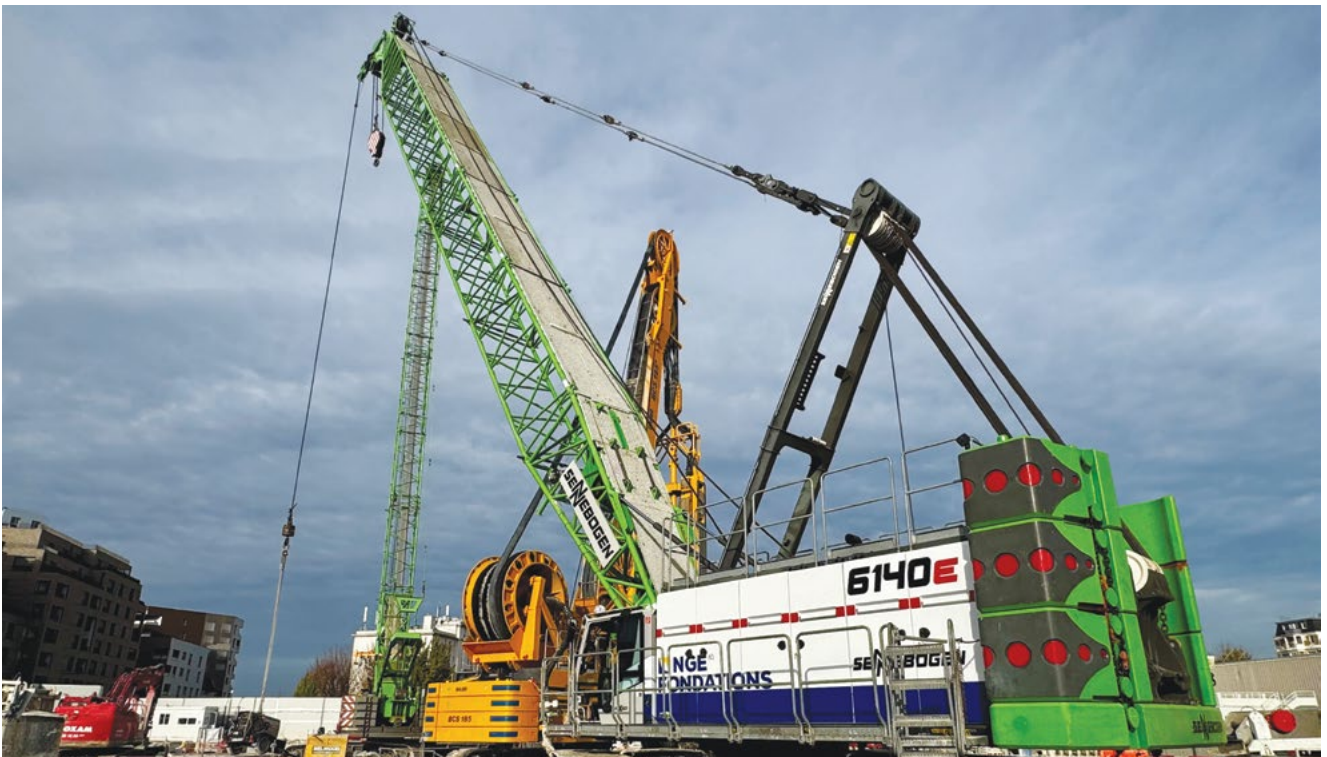
SENNEBOGEN duty cycle cranes during the construction of the entrance shaft for the tunnel boring machine (TBM) – the 6130HD with diaphragm wall grab in tandem with a hydro cutter and the 6140HD during heavy-duty lifting.
