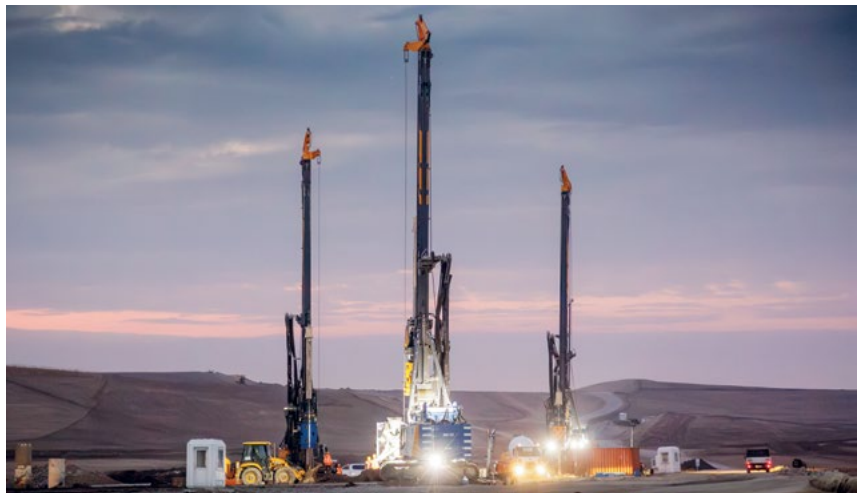
A whole fleet of Bauer rotary drilling rigs, pile drivers and mixing plants is being used for the new high-speed rail line in Central Anatolia.
