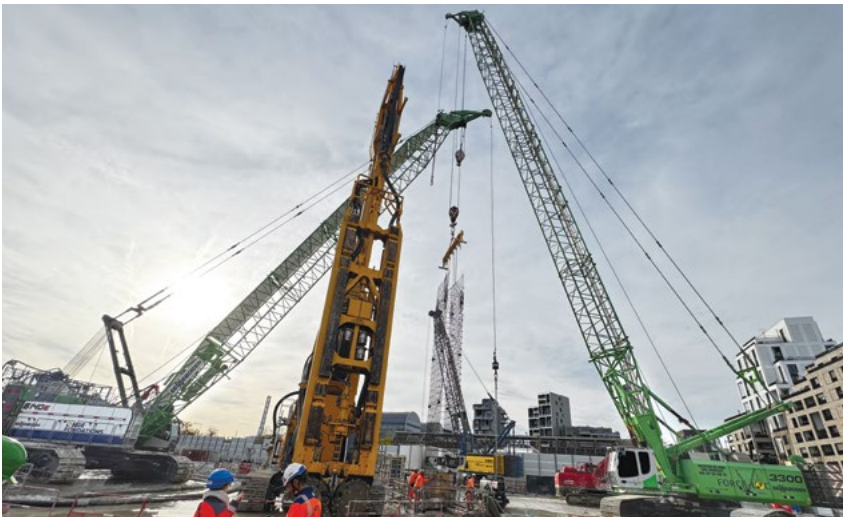
The SENNEBOGEN 3300 crawler crane from FORCE-LOC is used to assemble the reinforcement cages for the service structure for the TBM.
