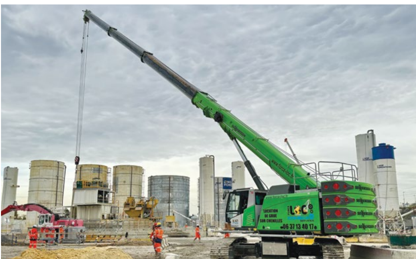
The SENNEBOGEN 673E crawler crane supports the concreting work, the preparation of the reinforcement cages, and various loading tasks at the Les Grésillons train station construction site in Gennevilliers.
