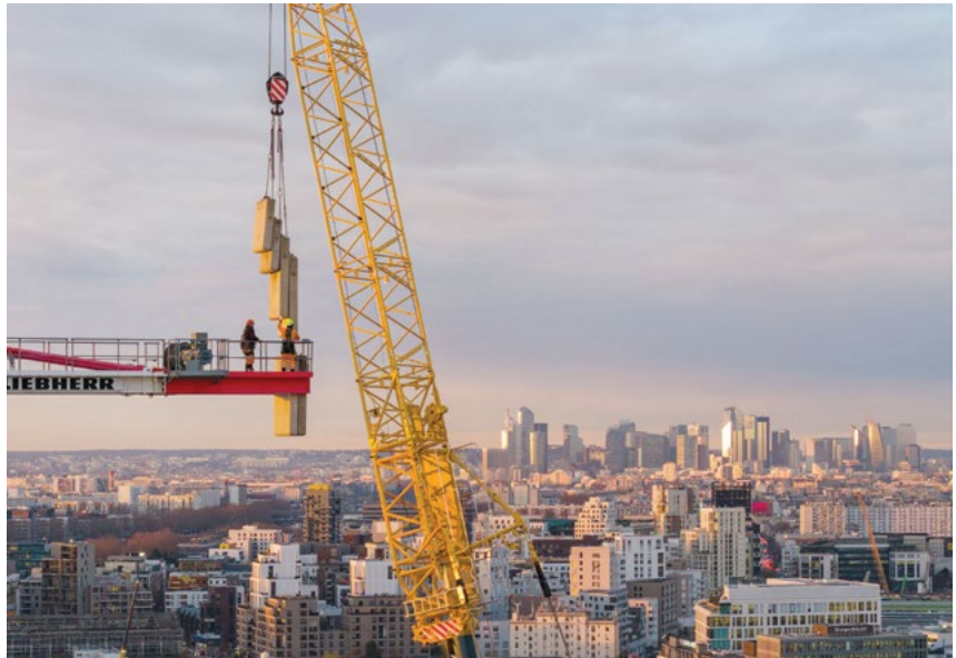
At a height of almost 80 m, the fitters hang four ballast blocks of the construction crane on the hook block of the LTM 1400-6.1.
