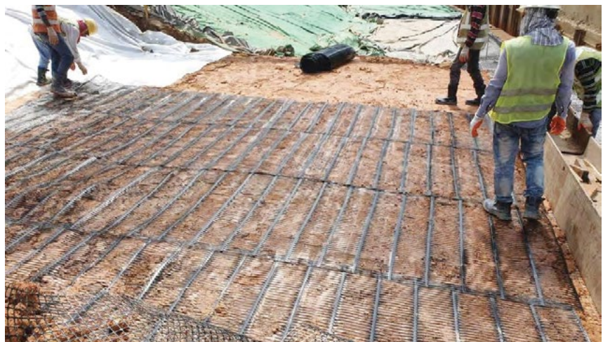
Figure 4: Laying of the unrolled geogrid before commencement of the work to build the geogrid-reinforced, soil bio-engineered slope.
