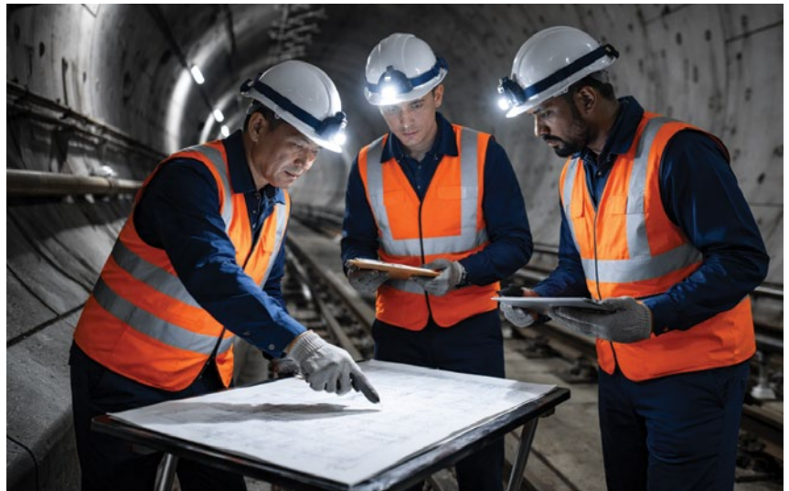
Engineers reviewing drawings during night-time works within an underground rail environment. Image: Daniel Woods.
