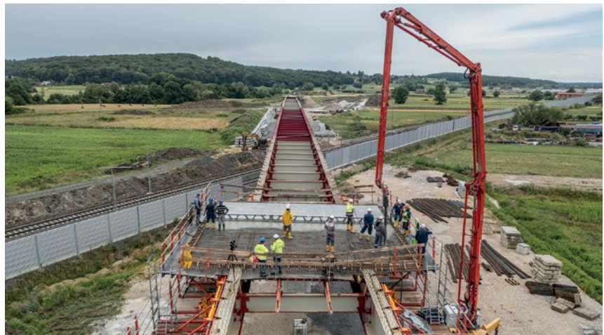
As the VCT Composite Track is moved beneath the superstructure and does not require any supports or carriageway penetrations, work can be carried out above without any hindrances. This simplifies and speeds up processes.
