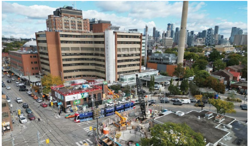
Toronto Western Hospital Noventa Energy transfer station. Image: R V Anderson Associates, 2025.
