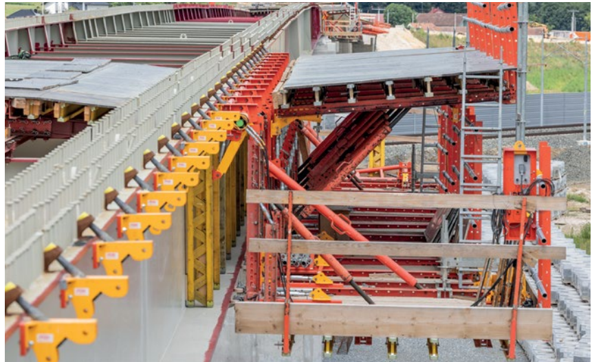
The VCT Composite Track runs beneath the superstructure and does not require any formwork carriage supports, which results in a higher quality of carriageway slab and simplifies and expedites construction processes. This is also made possible by a hydraulic drive.
