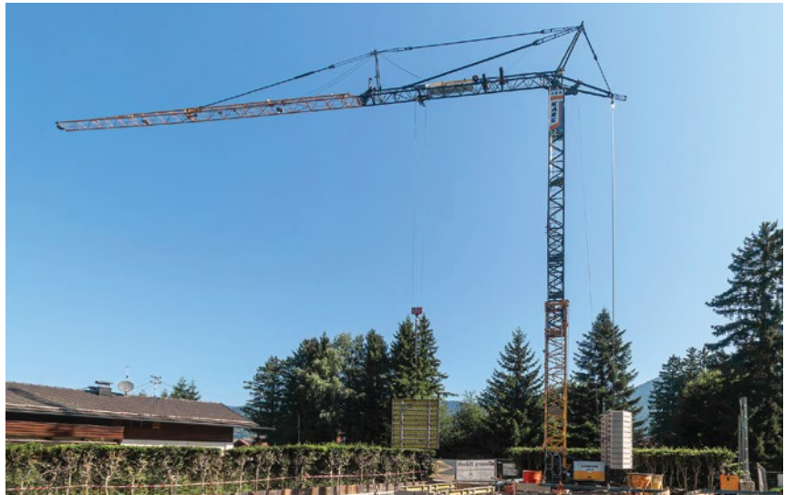
The new Liebherr 43 K is being used in the construction of a residential home with an underground garage in Rottach-Egern, Germany.
