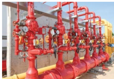
Foam system manifold.
