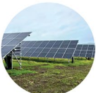
Ground Mount Solar
