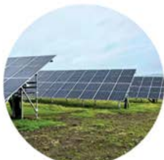
Ground Mount Solar
