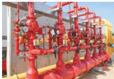
Foam system manifold.
