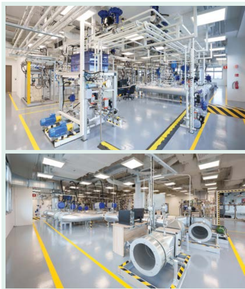
The EETF houses comprehensive industrial systems including pumps (top) and fans (below).
