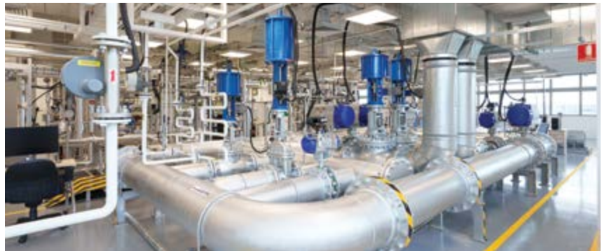
SIT's recently established Energy Efficiency Training Facility (EETF) features authentic, fully operational industrial systems. Image: SIT & Keng Photography.
