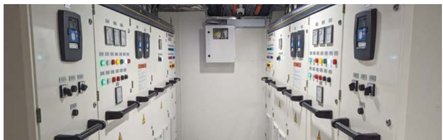
The main switchboards inside an Electric Dream ferry. Image: Danfoss.
