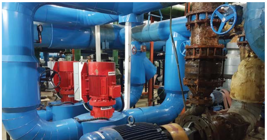
Armstrong Fluid Technology's Design Envelope pumps installed in Financial Park, Labuan.
