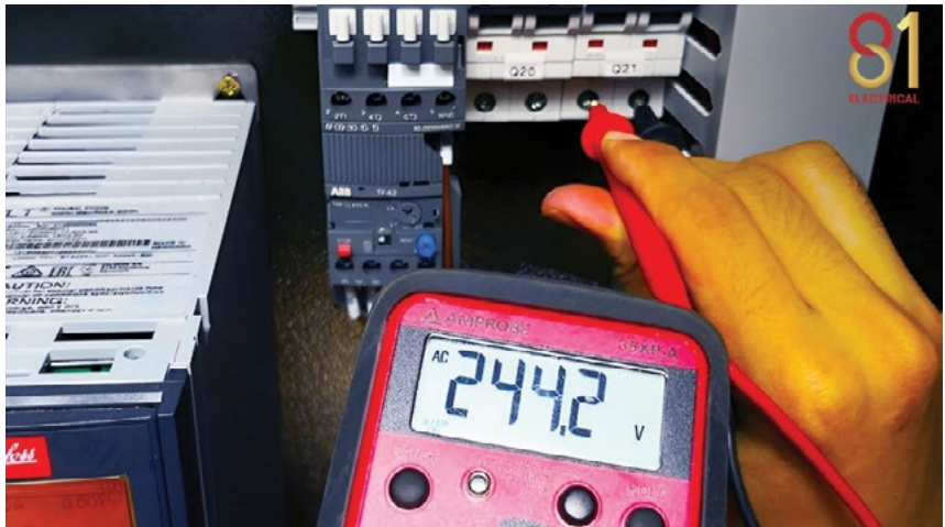
The control panel automation services from 81 Electrical will benefit many types of industries.
